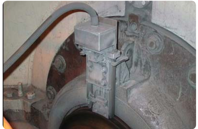
Fig. 5. Pendulum probe installation.
