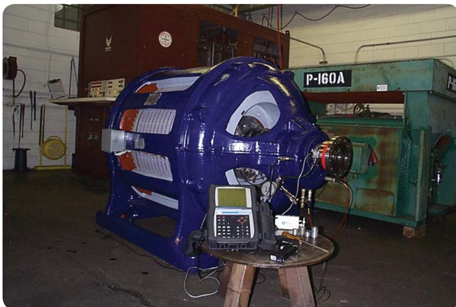
Fig. 1. Trim balancing 1 250 HP electric motor with CMVA 60 SKF Microlog data collector.
