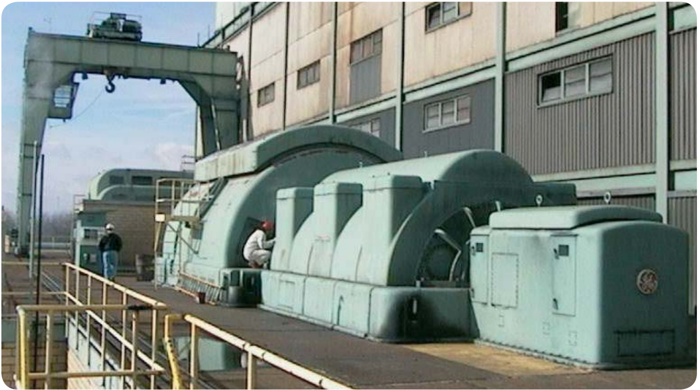
Figure 2. A Steam turbine generator train.
