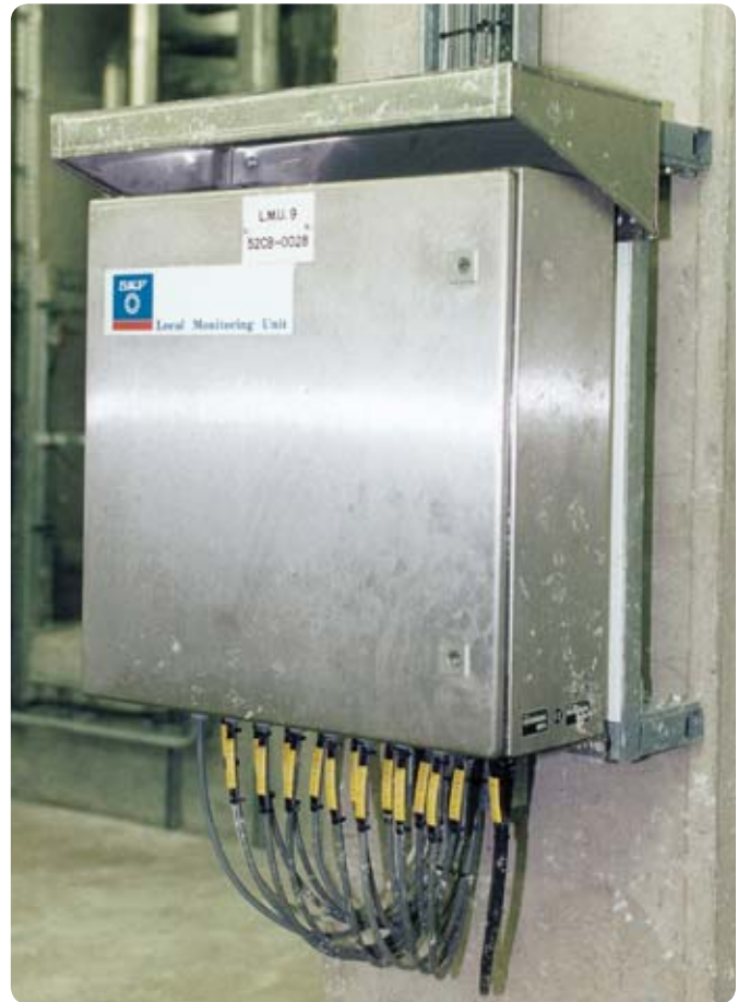
Fig. 2. Local monitoring unit (LMU).
