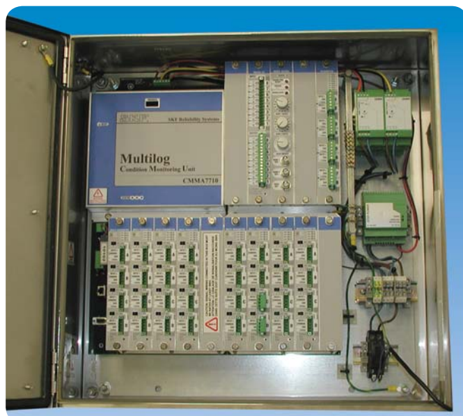
Figure 1. The SKF Reliability Systems Condition Monitoring Unit (CMU).
