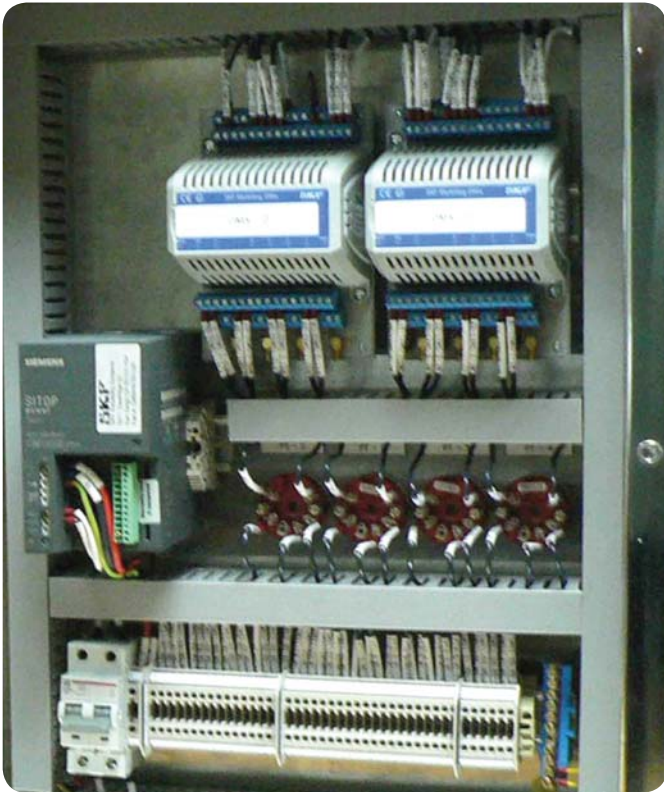
Figure 10. SKF Multilog DMx and PR5333D transmitters (in non-IS application).
