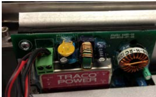
Figure 2 - 1. 24 V DC Power Supply Terminals.
