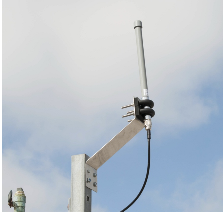
Figure 5 - 8. External Antenna Mounted to Pole.
