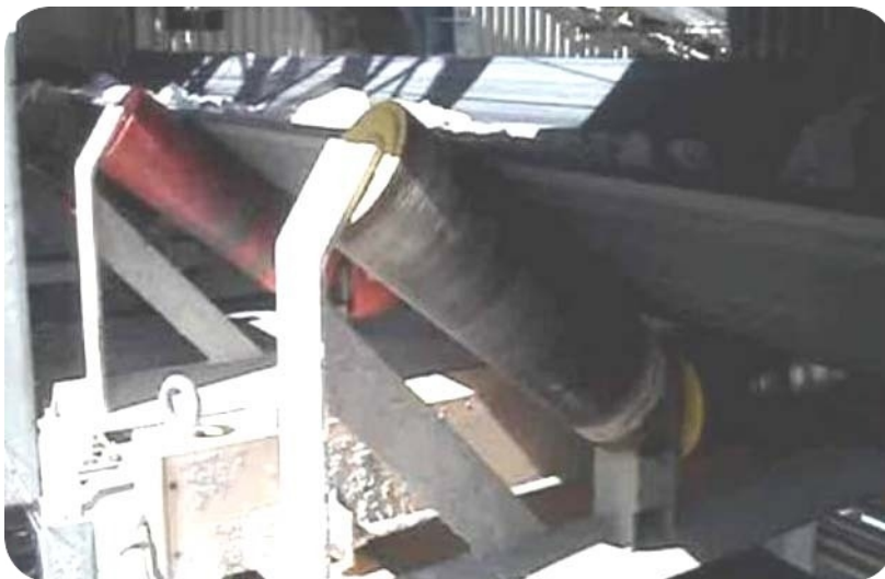
Figure 11 – 1. Conveyor Idler Rollers.
