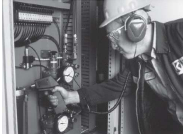
Figure 7. Detecting a Leak.
